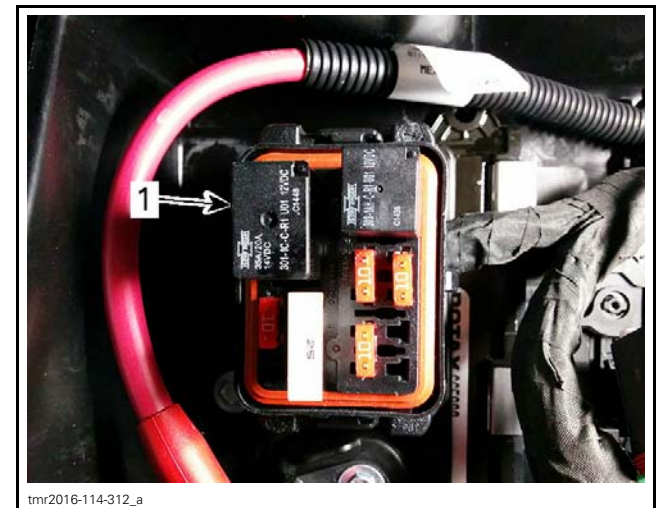
1. R1: Radiator cooling fan relay
